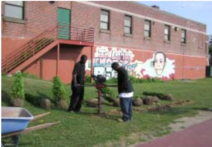
Two workers from Resource Services prepare the planting holes for the arbor vitae using a soil auger. BJ's mural is in the background.
